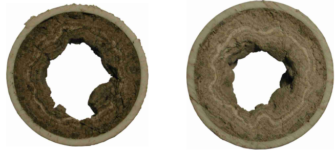
Cooling water pipes after less than one year's operation without filtration
